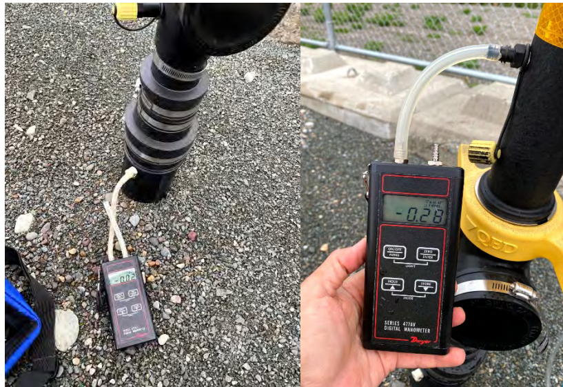
Photo 1 - Negative Pressure Maintained at the Wellhead by the Solar Powered Fan
