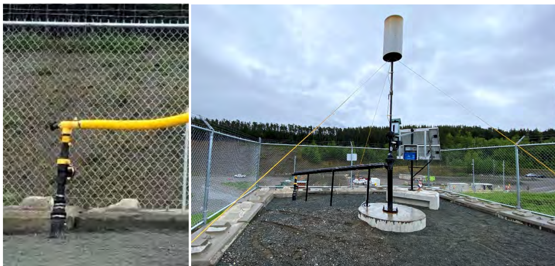
Photos 1&2 - QED Precision Wellhead (left) and Solar Spark Flare at the Thornhill Landfill (right)
