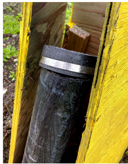
Photo 3 - Source of Air Intrusion into the Gas Collection System Identified and Fixed
