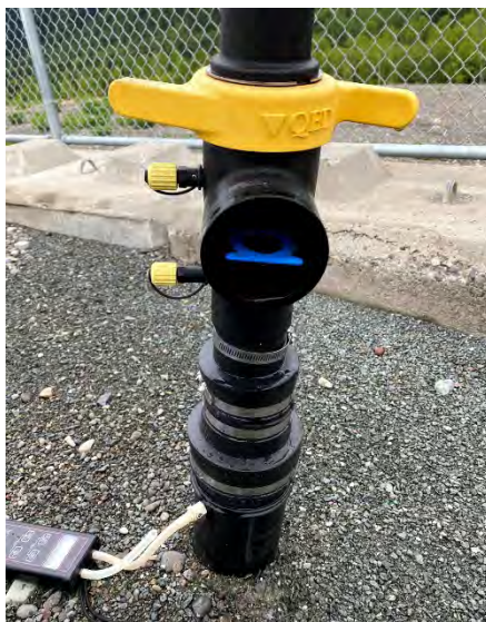
Photo 2 - Orifice plate Replaced from 1.25 to 1.4 Allowing Lower Head Loss Through the Wellhead
