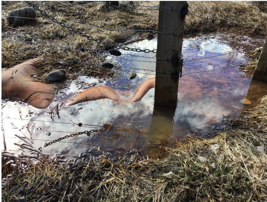
Photo 5: Kitwanga Landfill leachate breakout near northwest corner of landfill, looking south, April 13, 2022
