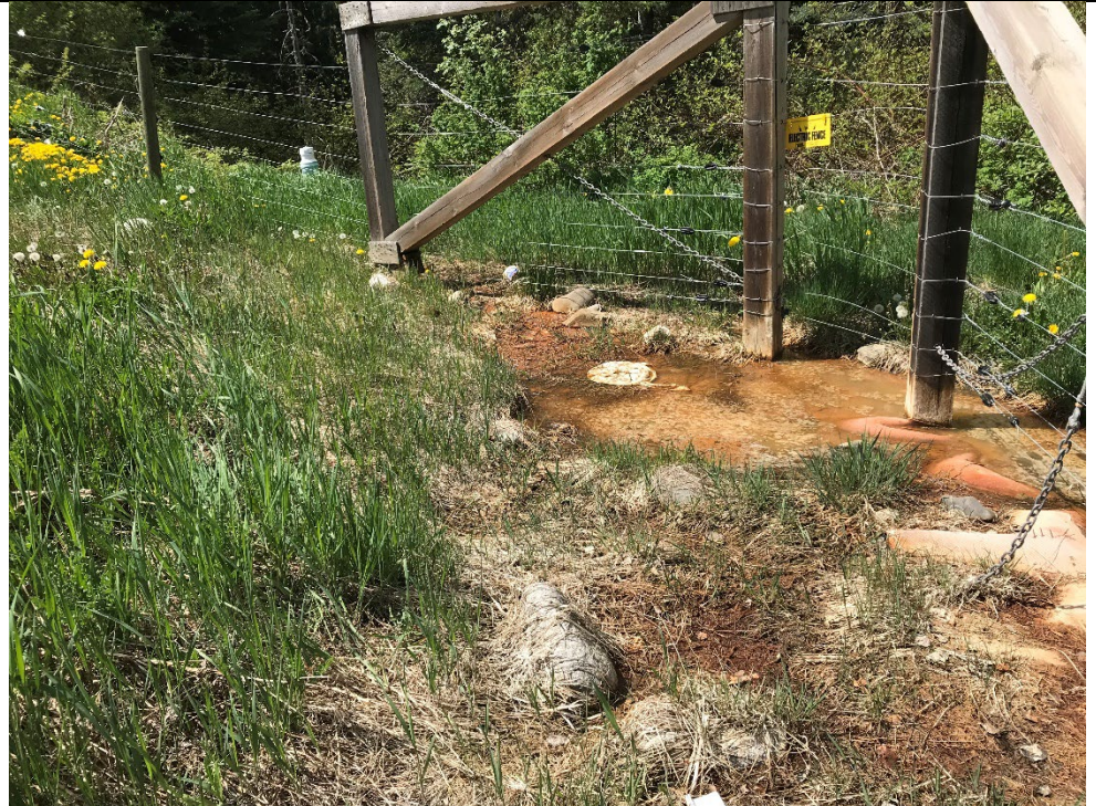
Photo 1 – Leachate breakout at the toe of the slope in the northwest corner of the landfill
